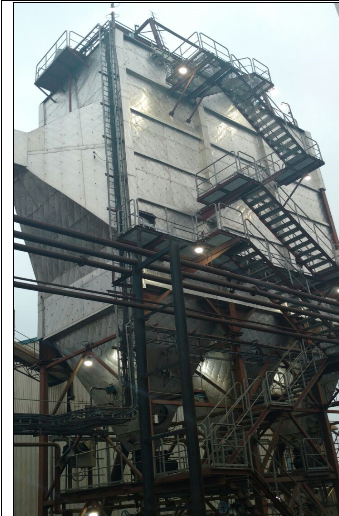
Electrostatic Precipitator attached to Stack
